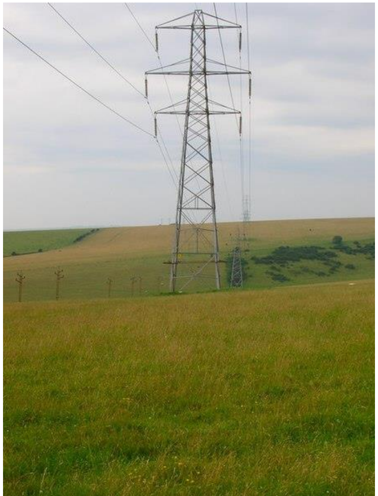
Electricity pylons in West Sussex, UK. Photo from Geograph/ Wikimedia Commons
